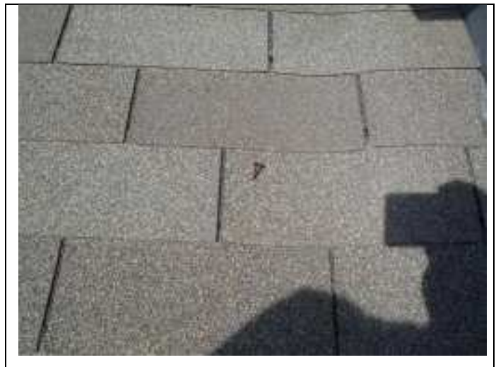
Sample of exposed nail in the roof
