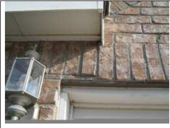
Sample of exterior brickwork crack
