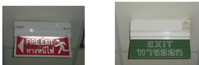
Figure 3 Fire Exit and Evacuation Route Signs of Mahamakut Building
