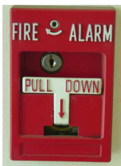
Figure 1 Fire Alarm Pull Stations of Mahamakut Building
