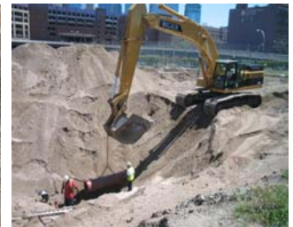
VCP Sanitary Sewer
