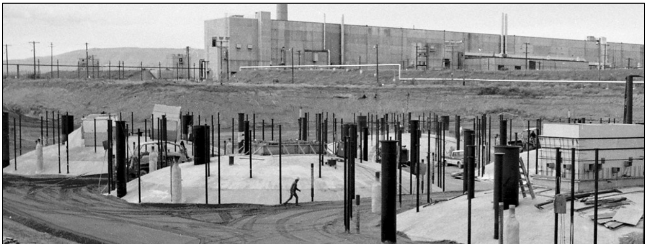
Construction photo, scanned by MSA IM Visual Services for Washington River Protection Solutions, of double shelled tanks at the 241AW tank farm.
