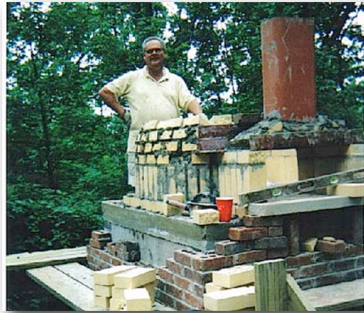
12.1. Refractory flue liner.
