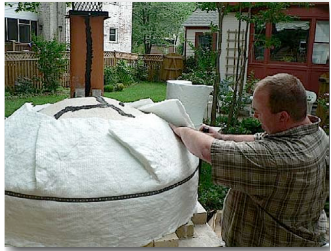
13.1. FB Blanket held in place with metal bands.
