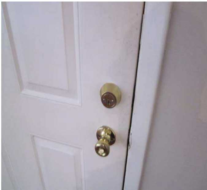
DEAD BOLT LOCK ON FRONT ENTRY DOOR NOT KEYLESS
