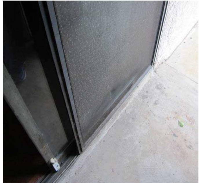
DAMAGED BACK SLIDING SCREEN DOOR
