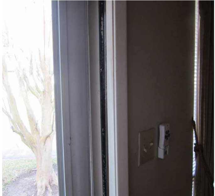
DAMAGED WEATHER STRIPPING ON FRONT ENTRY DOOR
