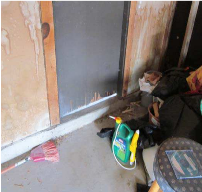
BADLY DAMAGED BACK EXIT DOOR OF GARAGE
