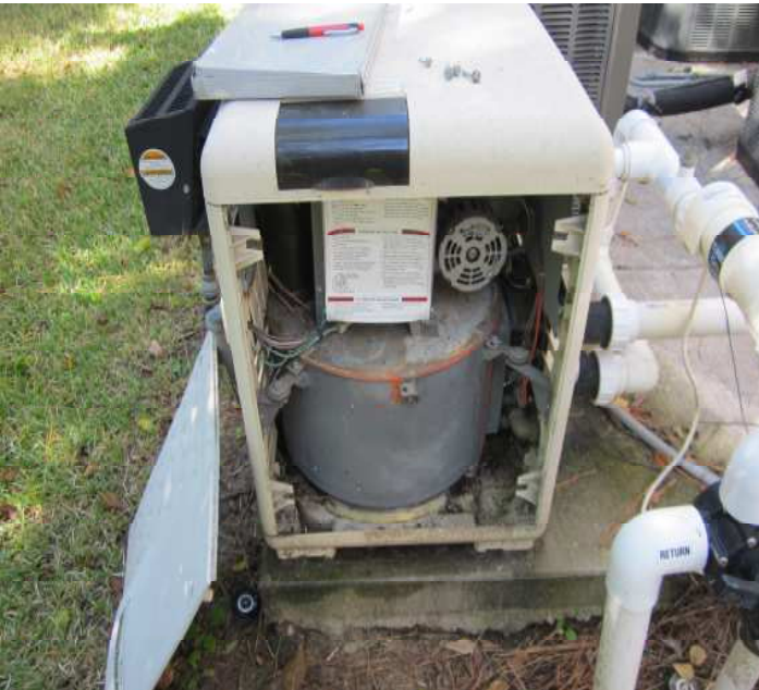
POOL HEATER BEGINNING TO RUST OUT
