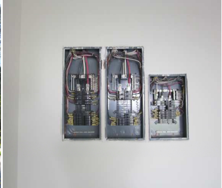
SUB-PANEL BREAKER BOXES INSIDE GARAGE
