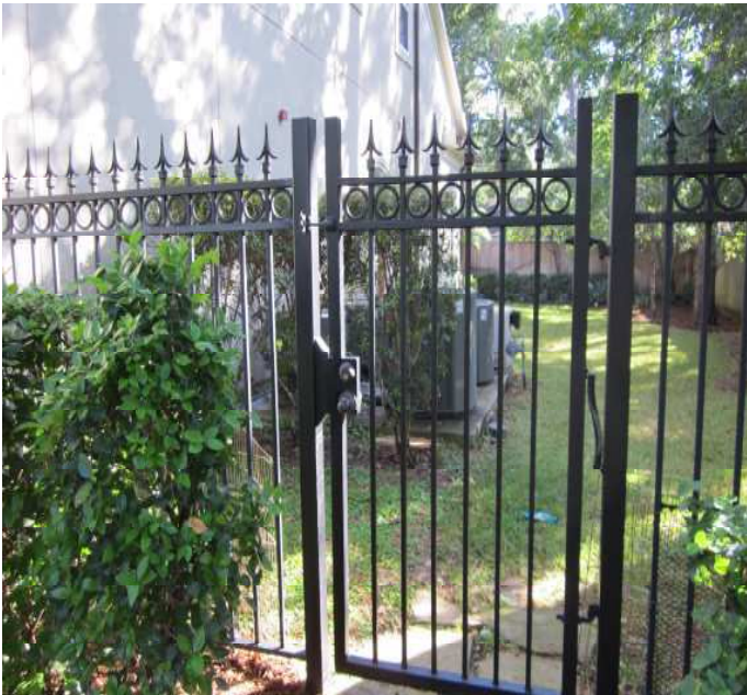
SOUTH SIDE GATE LOCK NEEDS REPAIR
