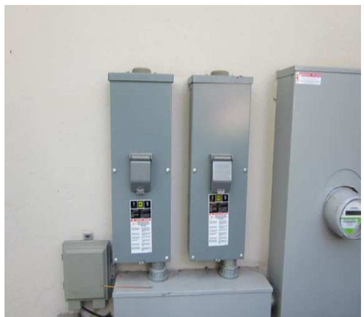
MAIN BREAKER BOXES ON OUTSIDE NORTH WALL
