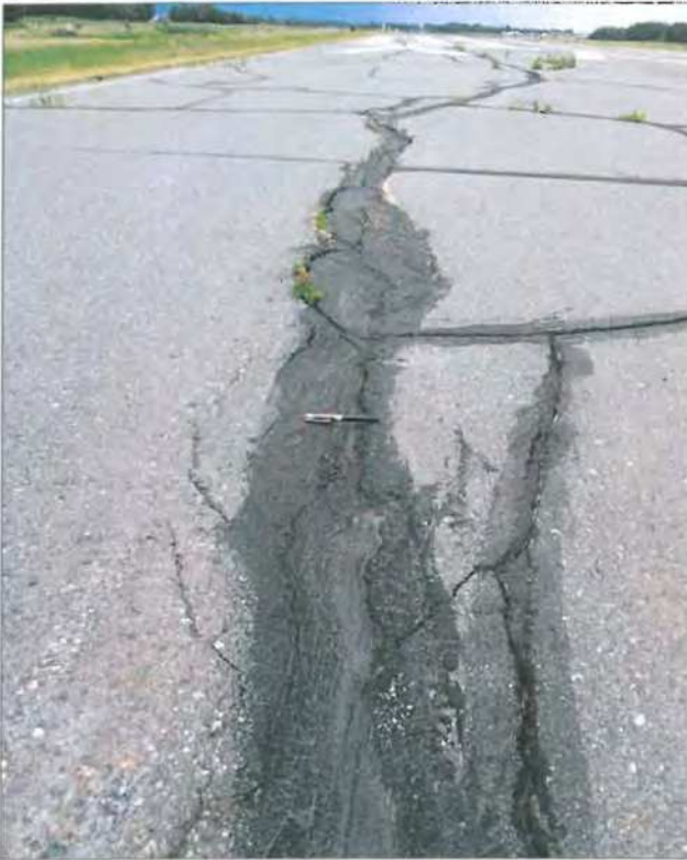
Photo 1: Longitudinal Crack, Displaced Threshold Area
