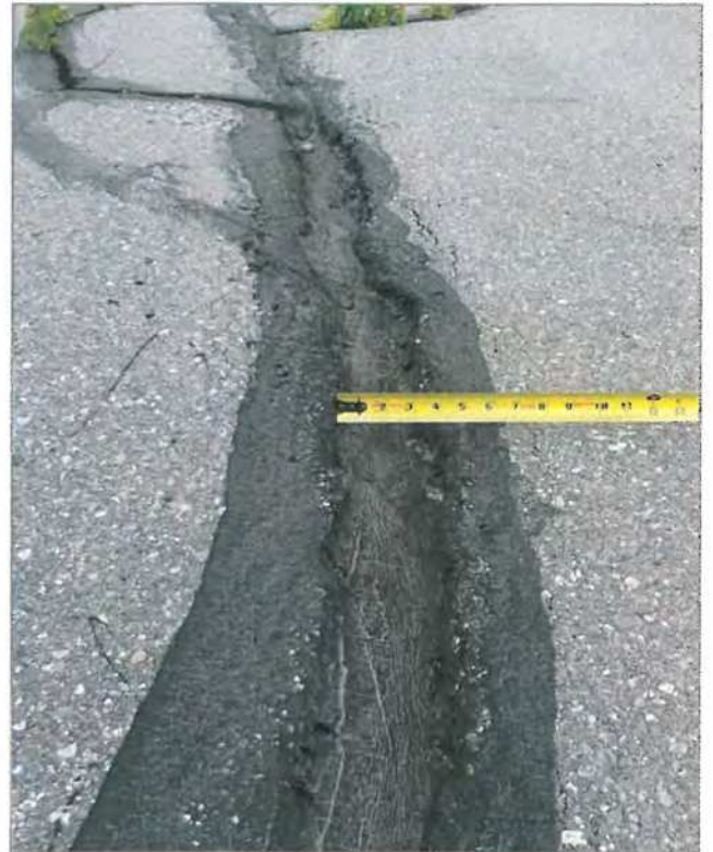
Photo 2: Longitudinal Crack, Displaced Threshold Area
