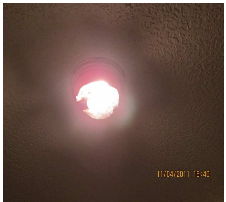
PHOTO NO. 20 BROKEN LIGHT FIXTURE IN UTILITY ROOM
