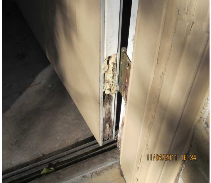
PHOTO NO. 18 DAMAGED BACK EXIT DOOR OF GARAGE
