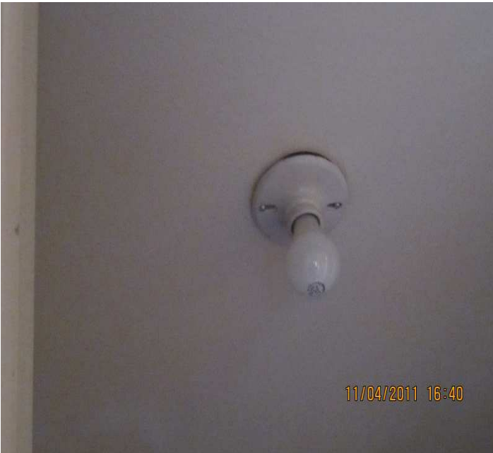
PHOTO NO. 19 CLOSET LIGHT FIXTURES MISSING GLOBES
