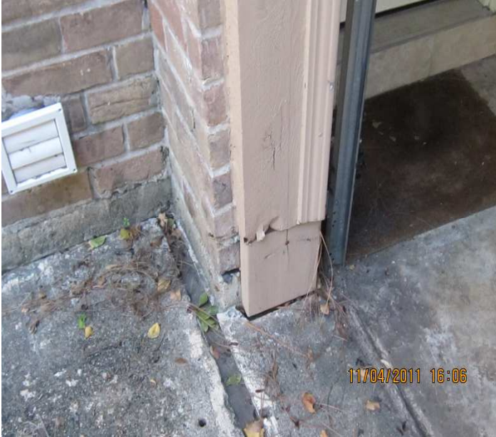
PHOTO NO. 13 ROTTING OUT VERTICAL GARAGE DOOR FRAME BOARDS
