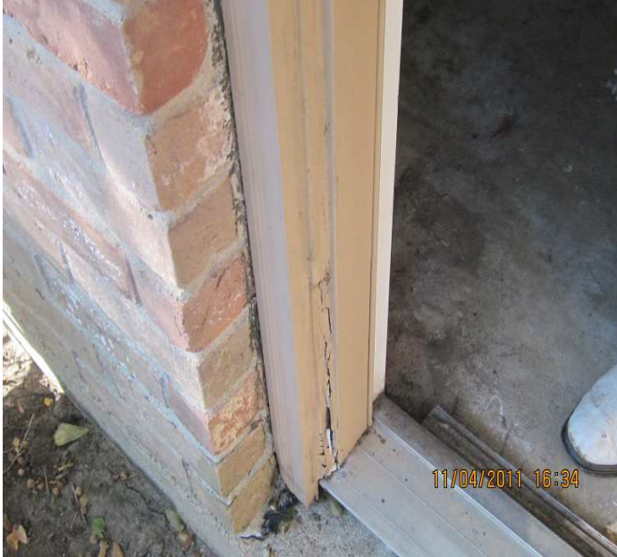
PHOTO NO. 17 DAMAGED DOOR FRAME AT BACK EXIT DOOR OF GARAGE
