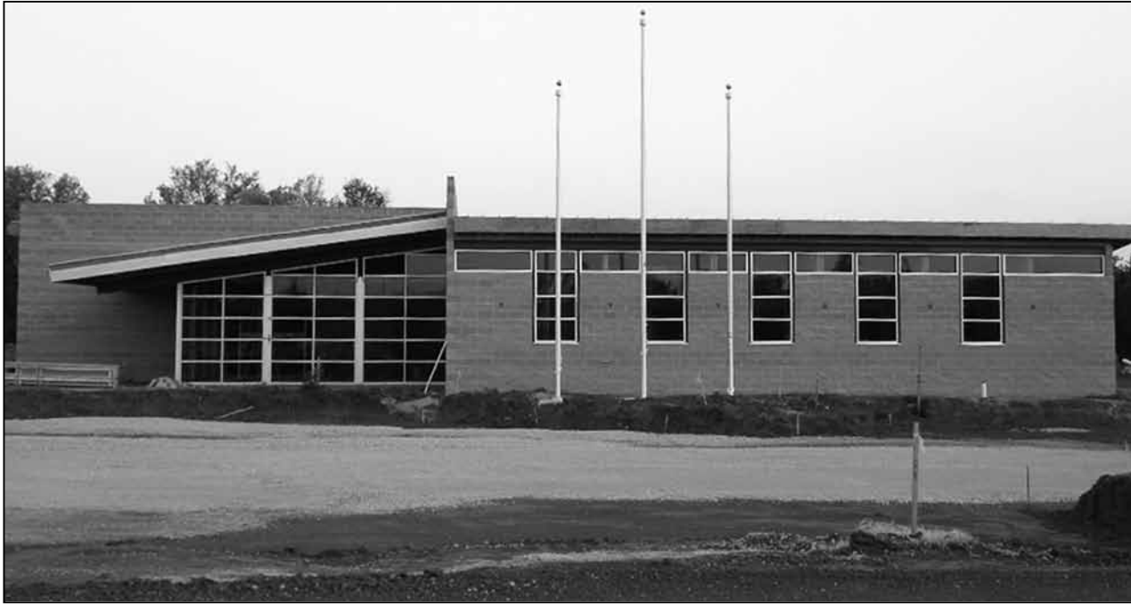
The Pawnee Nation Law Enforcement Center reaches the final stages in construction.
