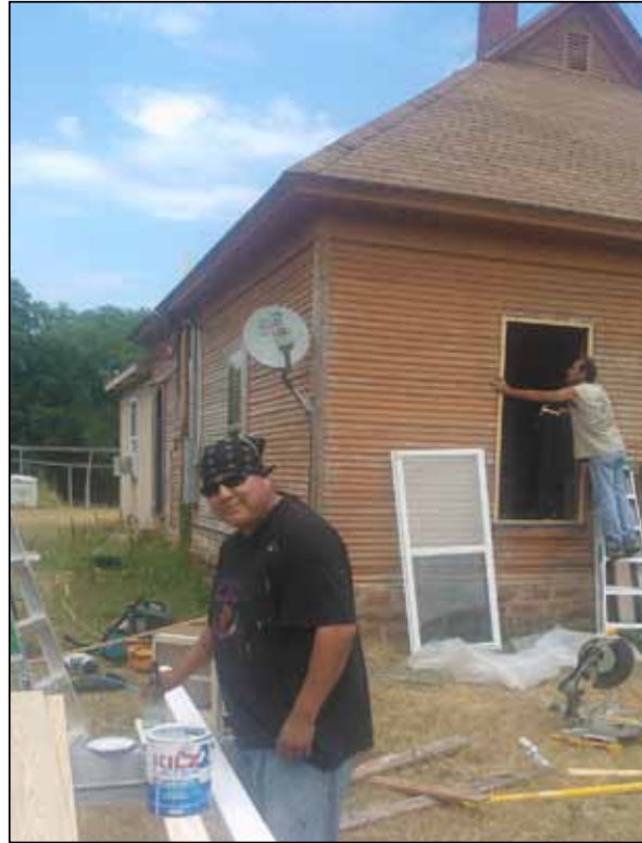
Dusty Eaves (front) prepares the new trim boards while Ronnie Cooper continues to reframe.
