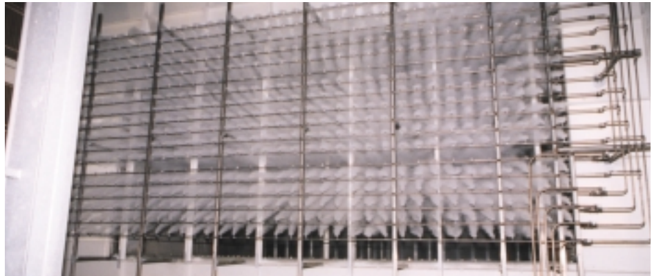
Gas Turbine Mist Cooling System
