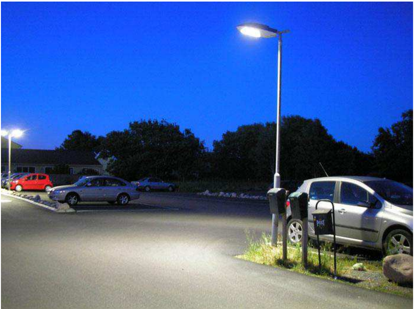
Figure 8: Parking lot Safety Lighting/LED technology
