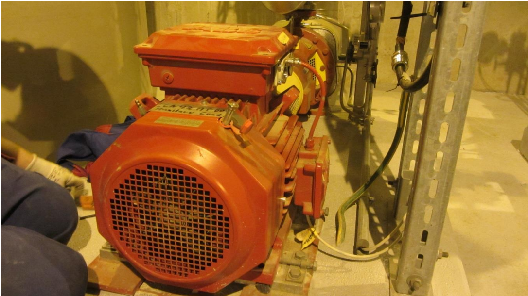
Figure 27. Some of the motors were only grounded through the incoming supply cable at the cable terminal box, like the 1LCN41AP001 (Cond Pp 1 AuxCondSys) motor in the picture. An additional grounding cable was connected to the case.
