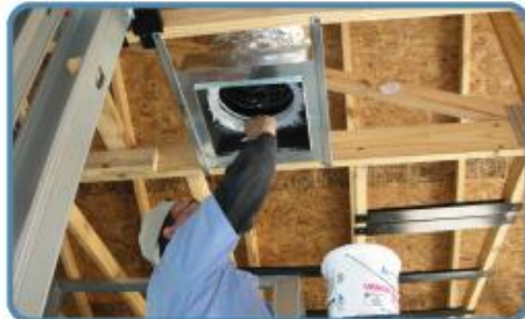
3. Perform a commissioning test to ensure the system is operating as intended.
