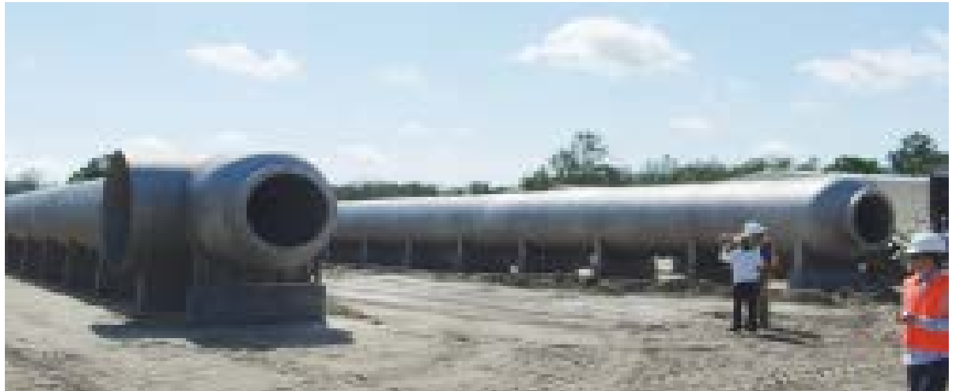
Picture above: Pipework for the hydrogen sulphide removal stage of waterworks.
