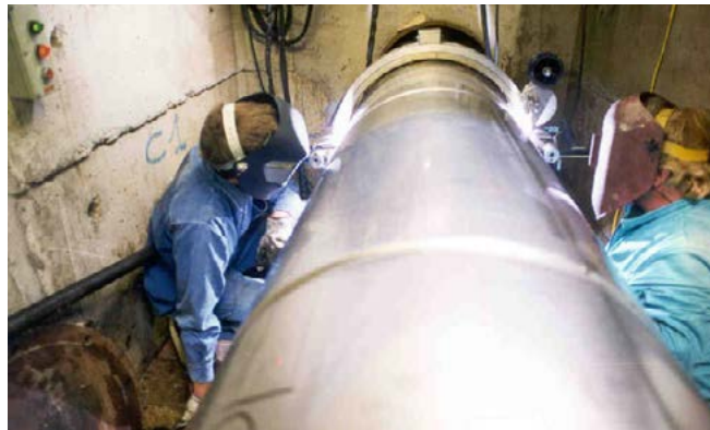
Stainless steel inserts as a repair solution for underground main supply lines.
