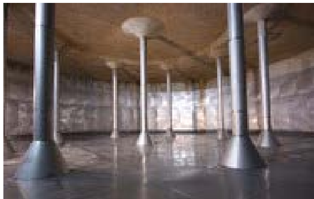
Stainless steel linings of concrete reservoirs. Source: www.forstenlechner.at
