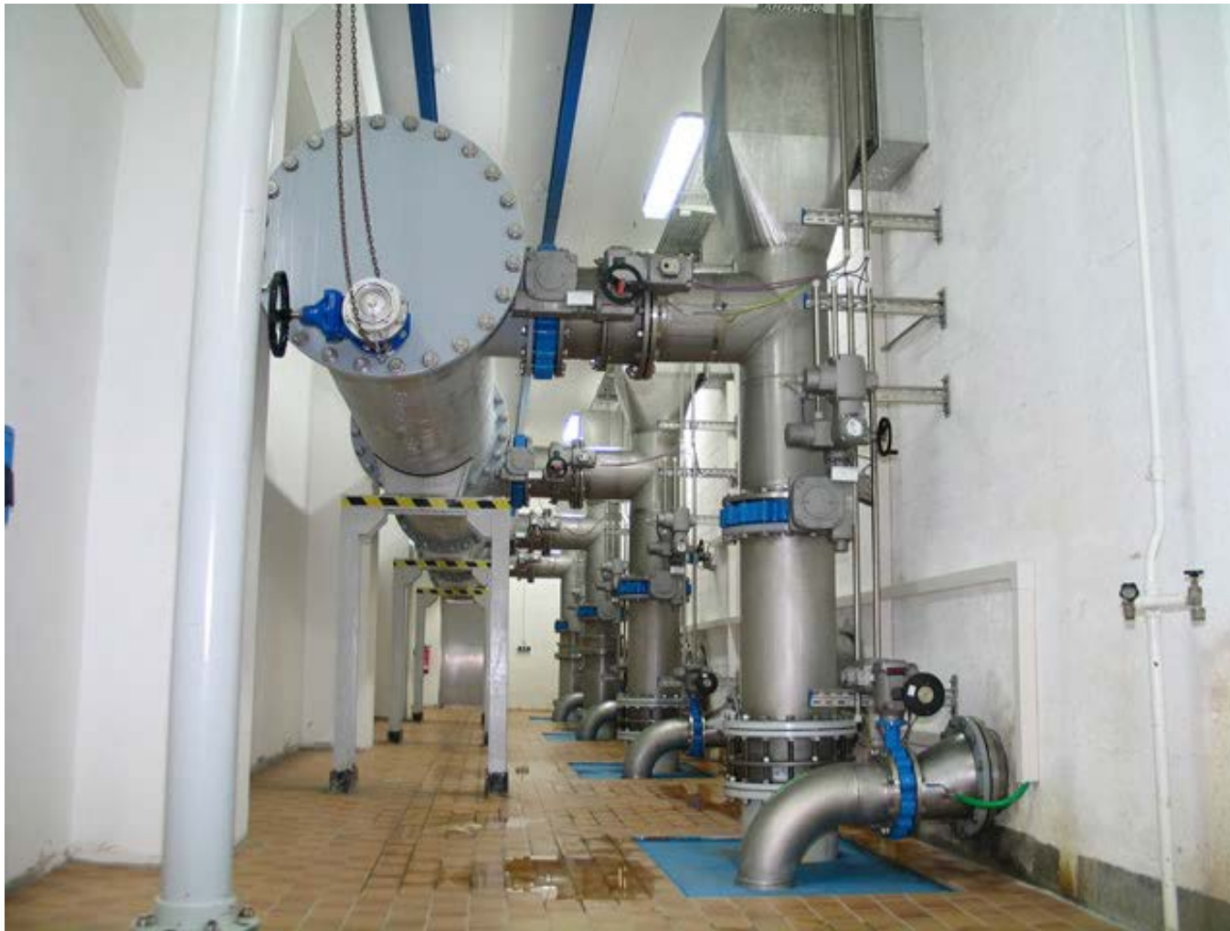
Stainless steel in municipal waterworks. Source: Schenke Anlagenbau, (Germany), www.schenke-anlagenbau.de
