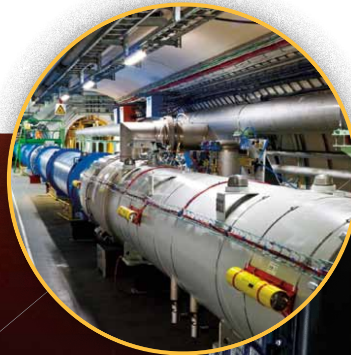
View of the LHC machine in the Switzerland tunnel. Photographs courtesy of the ATLAS experiment at CERN, Maximilian Brice
