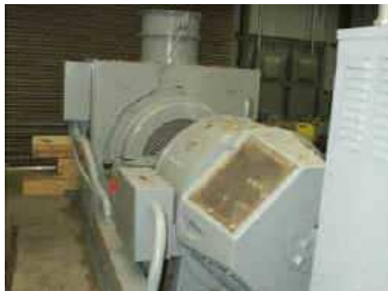
Figure 44. Electric drive system.
