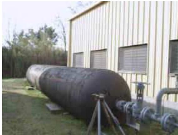
Figure 40. High pressure air storage tank.
