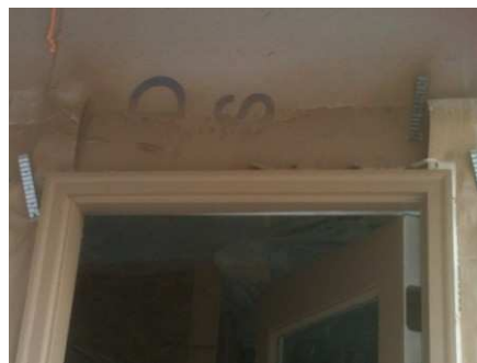
Incomplete flashing at top rear patio door
