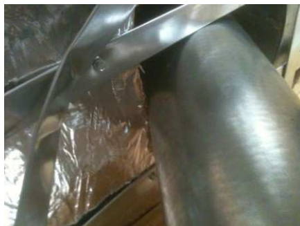
Heating unit flue vent pipe touching wood
