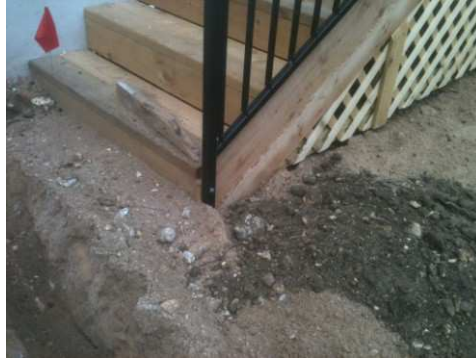
Soil-covered stair base and sprinkler flag (ill-advised)
