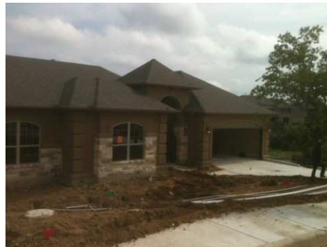
Irrigation and final grade not completed as of 3/27/12
