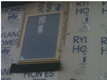
Incomplete window flashing rear left corner
