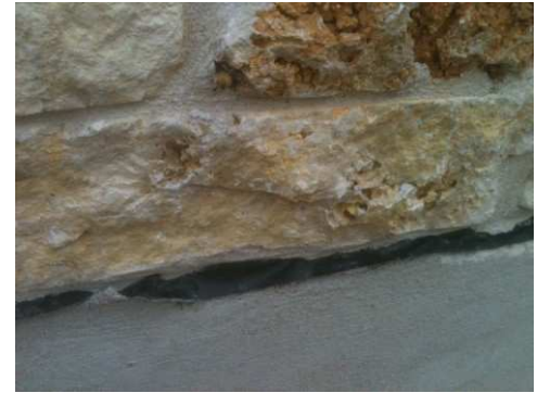
Moist stop protruding past lower course of stone
