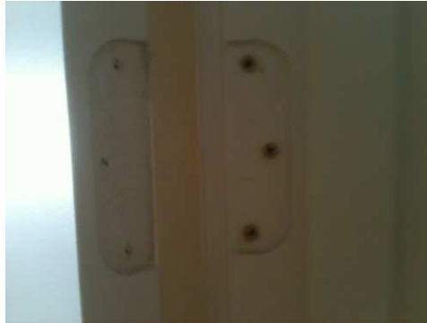
Missing hinge at garage water heater door (left)
