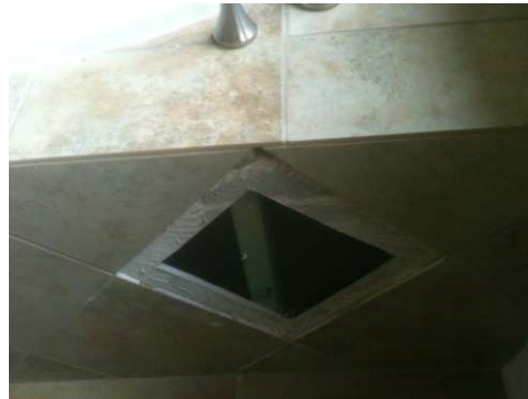
Missing tile and sheetrock at master tub skirt
