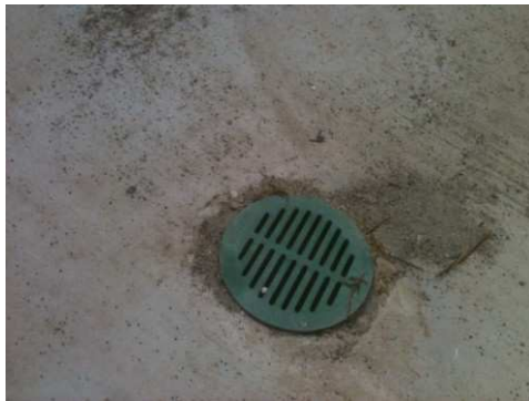
Drain grate too high for effective drainage in courtyard
