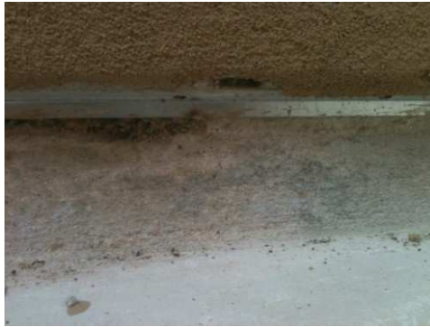
Courtyard weep screed needs work in some areas
