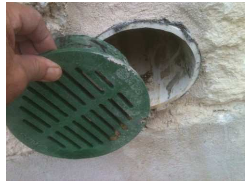
Drain grate not secured to drain terminus along left side
