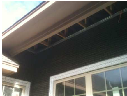
Incomplete soffit above front door
