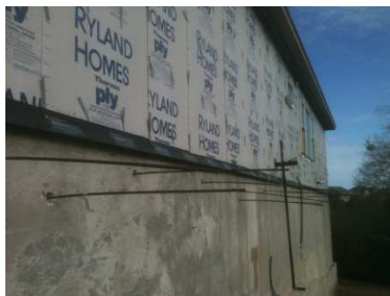
Post-tension cables not completed
