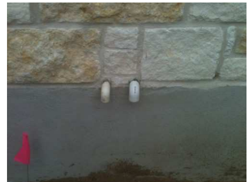
T&P terminus 12-15" above grade (should be 6")
