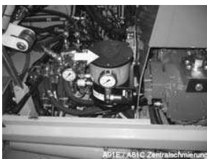
Central lubrication Regular checking of
