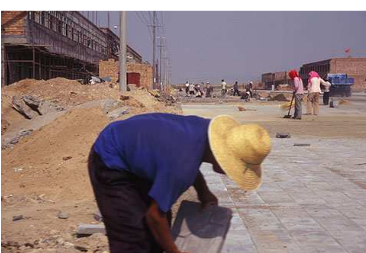
Construction has brought a wealth of new jobs to Hongsibao and the surrounding region.
