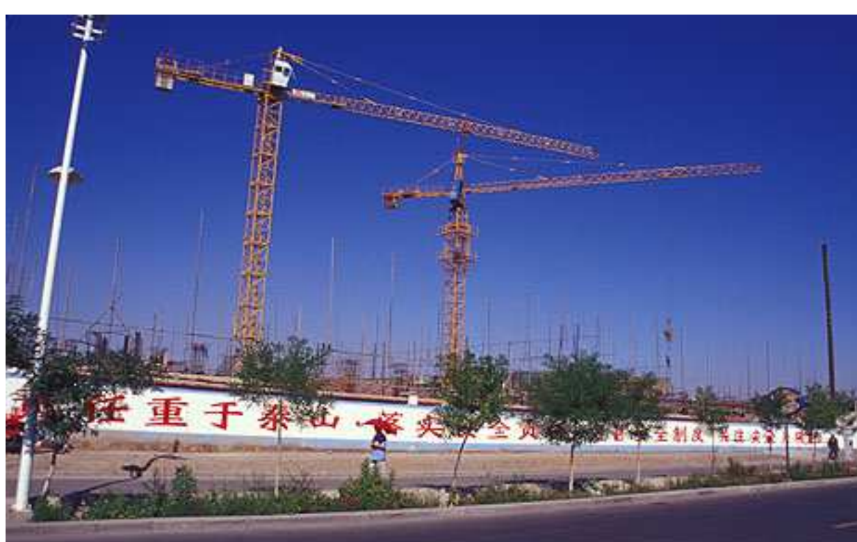
Cranes in Jiayuguan mark the rapid growth of the city, despite its problems with desertification.
