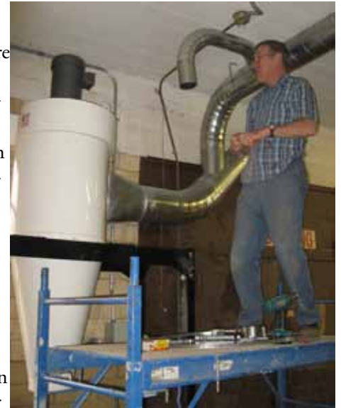
Br. Jude working to install the new dust collection system in the carpenter shop
