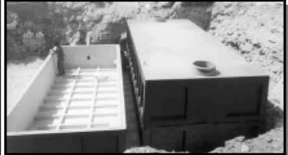
18,000 Gallon Precast Concrete Tank
