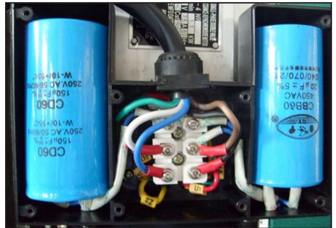
Figure 37. Spindle motor capacitors and wiring connections.
