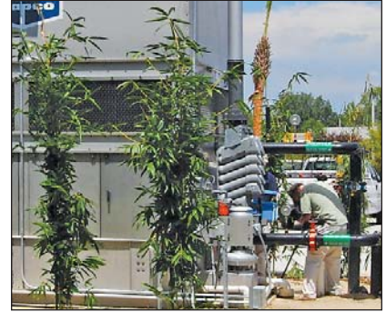
Closed Circuit Cooler Gainesville, FL USA
