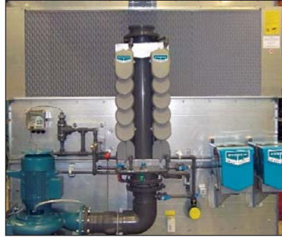
Closed Circuit Cooler Bruges, Belgium
