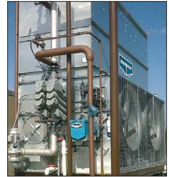
Evaporative Condenser Miami, FL USA
