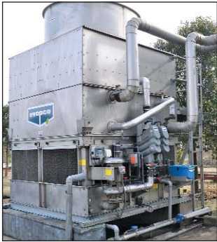
Closed Circuit Cooler Shanghai, China
