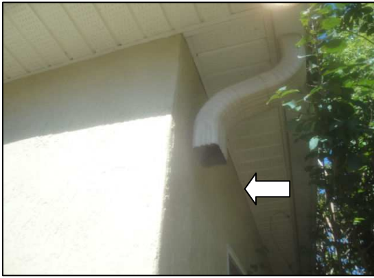
gutter not installed
