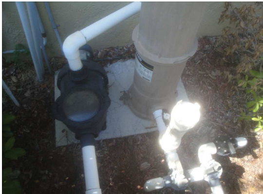
leaky seal at pump
