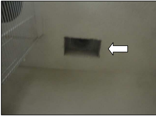
missing grill cover
