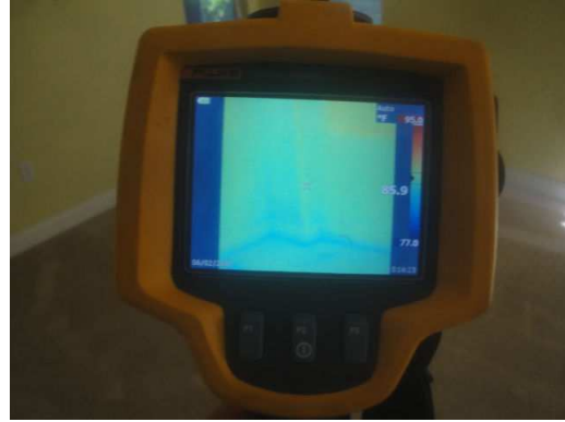
water intrusion at base
