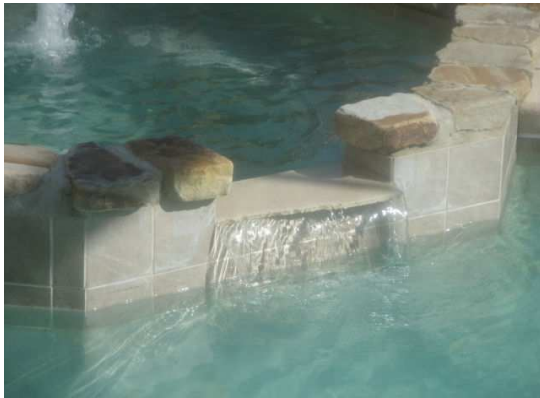
broken sill plate
