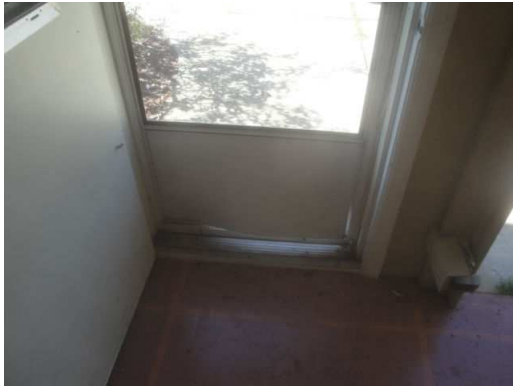
damaged storm door
