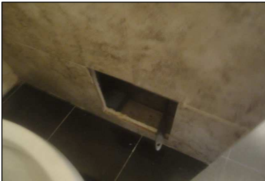
missing acces cover panel
