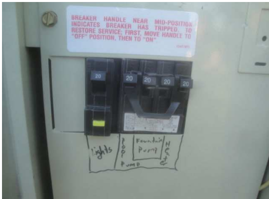
pool heater not on separate breaker
