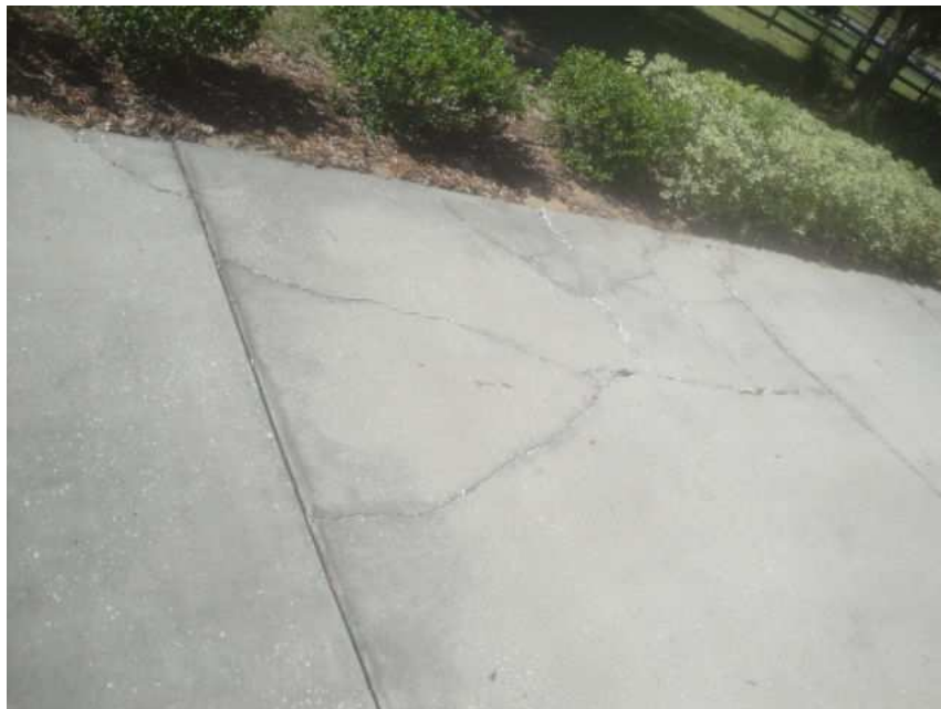
area requiring repouring
