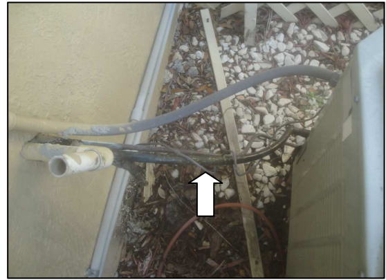
missing suction line insulation
