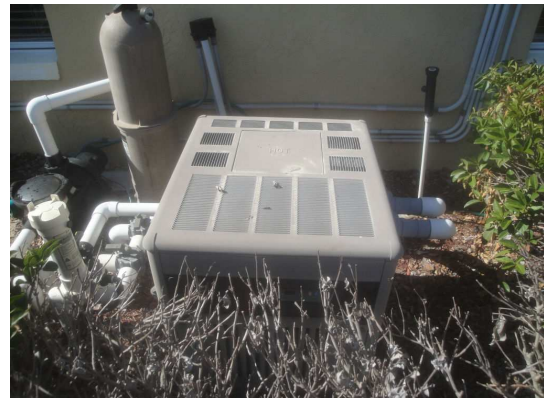
pool heater did not operate
