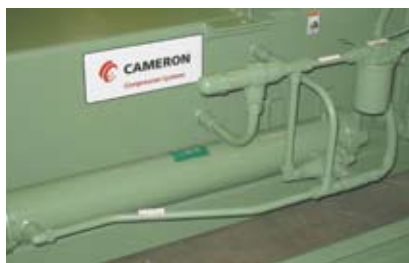
Self contained, low pressure lubrication system.
