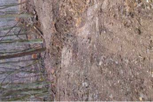
Skid road in process of being properly reclaimed. Note that it is smoothed and water-barred and berms on outside have been removed.
