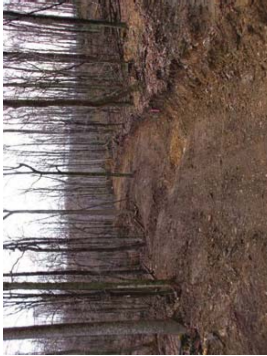
A good water bar. Note outflow end is open and proper construction angle across road.
