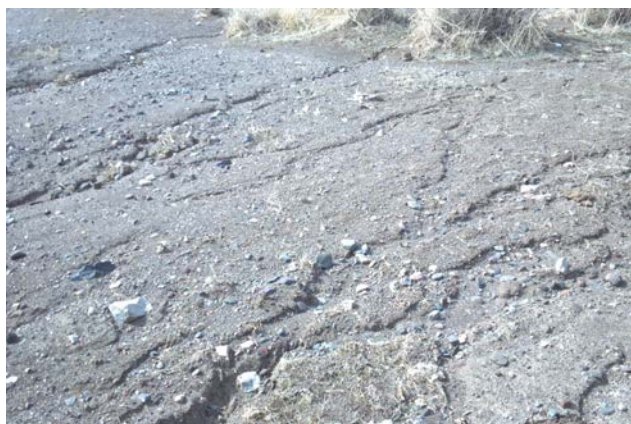
Sheet & Rill Erosion (Score = 0)
