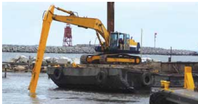
The RYC slip system is now deeper, thanks to the dredging done this fall.
