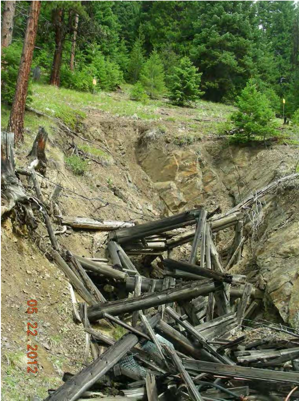
New Independence Crosscut, note FS property is behind signs above collapsed portal
