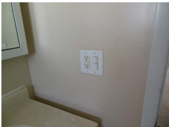
Replace with GFCI
