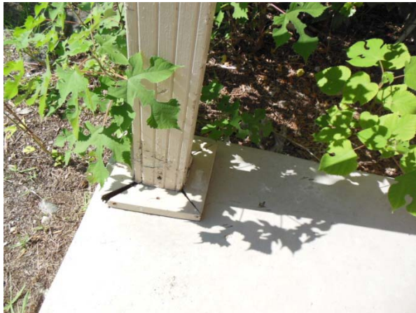
Remove rotted trim at base / inspect column
