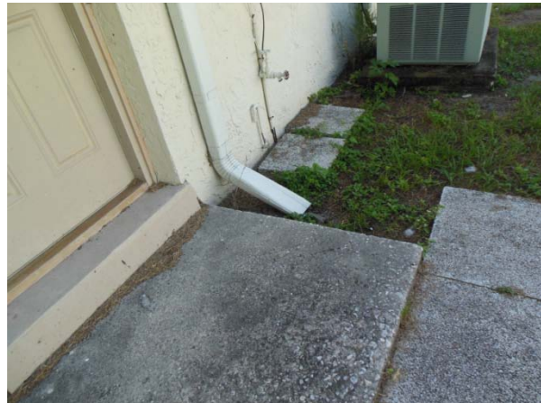
Replace damaged downspout extensions
