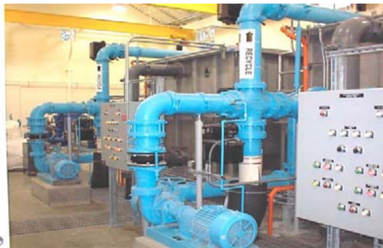
Vacuum DE Filtration Equipment (Courtesy of Separmatic)
