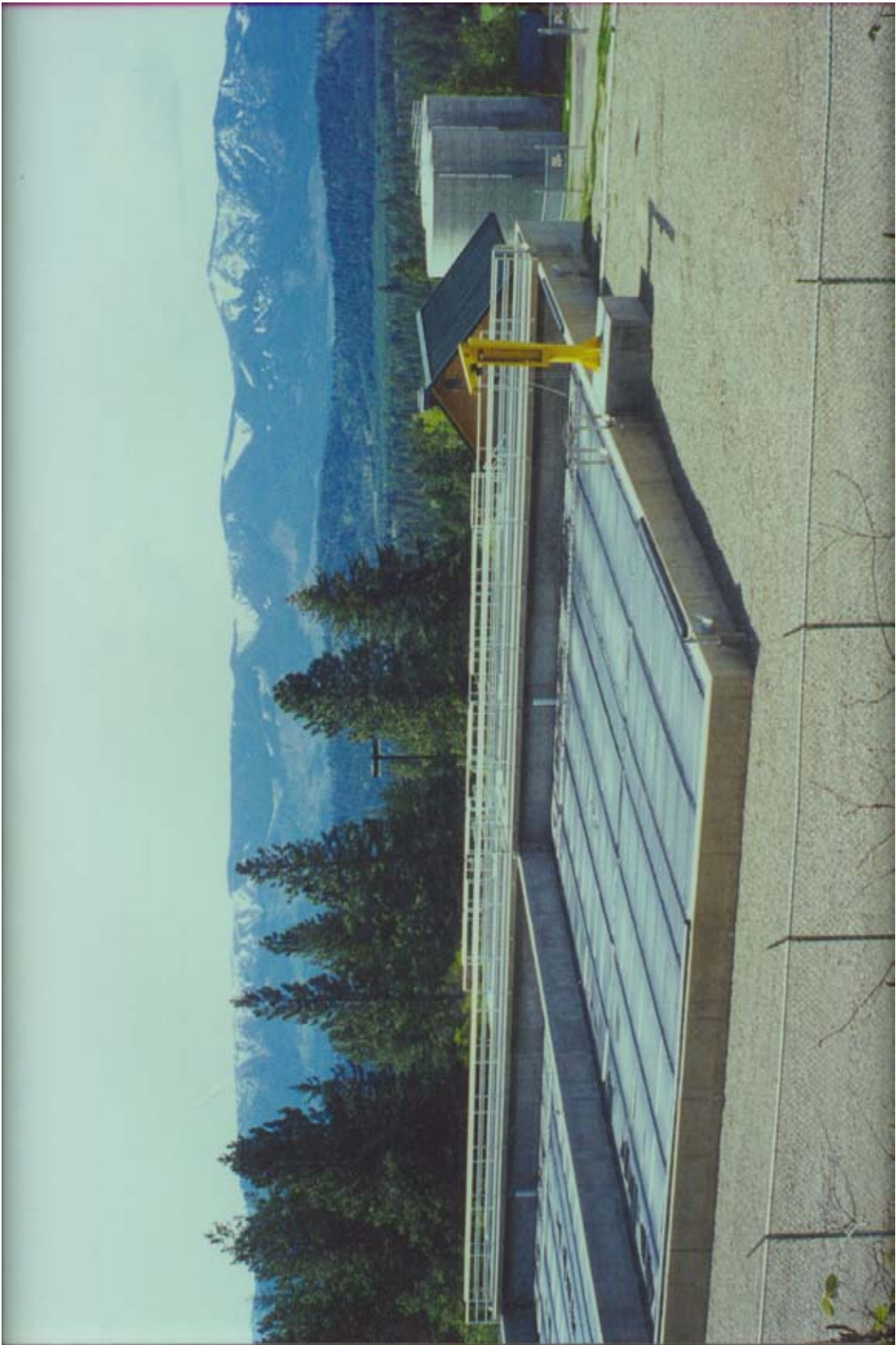
Figure 3-1. 1.0 MGD Slow Sand Filter at the City of Roslyn
