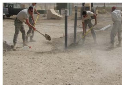
Electrician, EAs, and Heavy Operators work together to install conduit lines prior to concrete delivery for building foundation.
