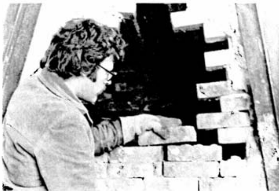
It took six weeks of hard work before Rocky Bivens was able to place the last brick on his kiln. Rocky, who built four smaller kilns before his major project, is delighted with the used roaster bricks he received from Inco.
