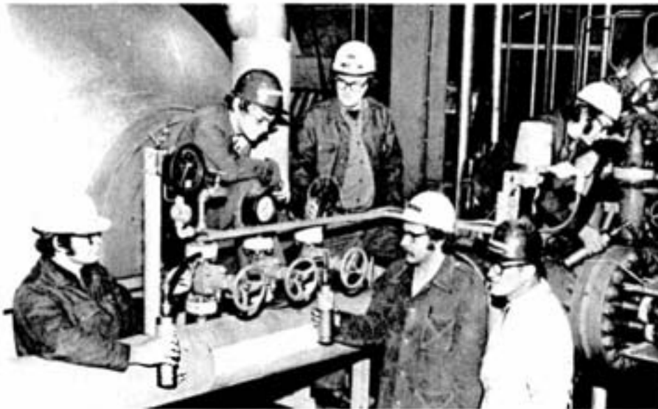
To a team from Port Colborne's research station fell the exacting task of leak-proofing the Copper Cliff nickel refinery. Climbing over this pipeline are John Gagnon, Rick Biederman, reactor supervisor, Al Shaubel, Bob McGowan, Peter Race, Bill Fordy, decomposer supervisor.
