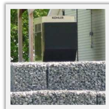
Elevated Emergency Generator
