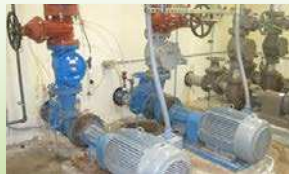
Booster Stations and Other Pumps
