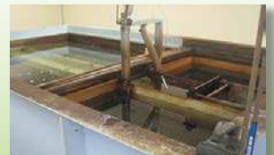
Drinking Water Treatment Plant
