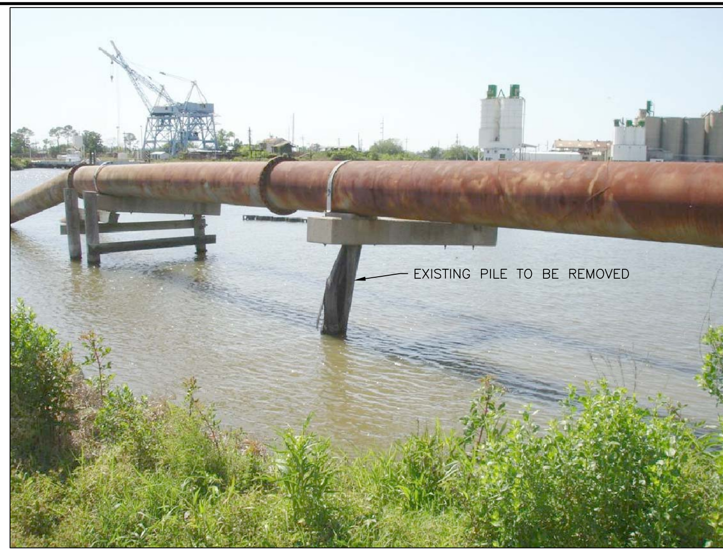
PHOTO — DAMAGED PIPE SUPPORT
