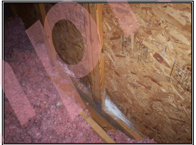
Miscellaneous photo of mold growing at other areas at the base of the right gable end siding.
