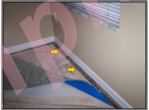
Photo 4- Decay damaged section of the moist tack strip in the right front bedroom.
