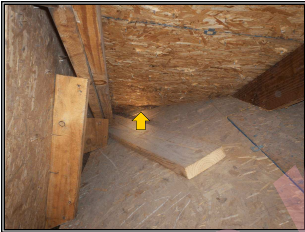
Photo 3- Wood decay at a section of roof sheathing below the base of the valley right of the garage.
