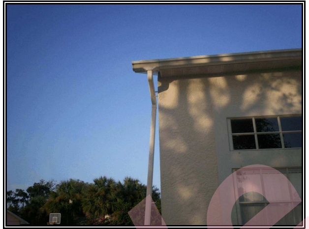
Photo 8- The loose rain gutter down spout at the left front corner of the house.
