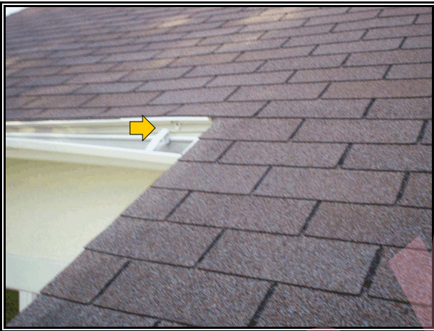
Photo 9- The disconnected run to the front of the living room.
