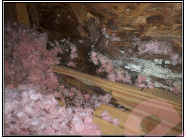
Photo 2- Another decayed section of the right gable end siding above the hall bath wall below.
