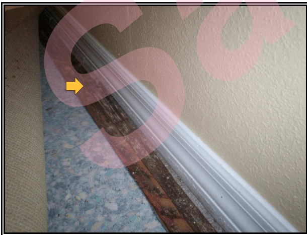
Photo 5- Decay damaged and slightly damp carpet tack strip at the front of the living room.
