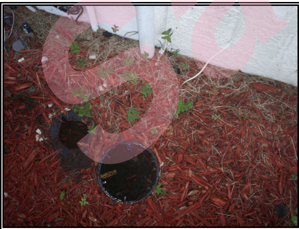
Photo 11- The missing caps at the domestic and lawn sprinkler shut off valves right of the home.
