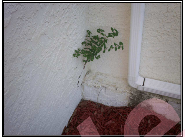
Miscellaneous photo of the plant growing in the crack at the left side of the home.
