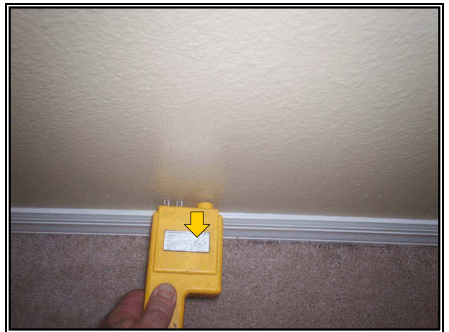
Photo 6- Increased moisture at the wall below the dining room window. The tack strip below is stained as well.
