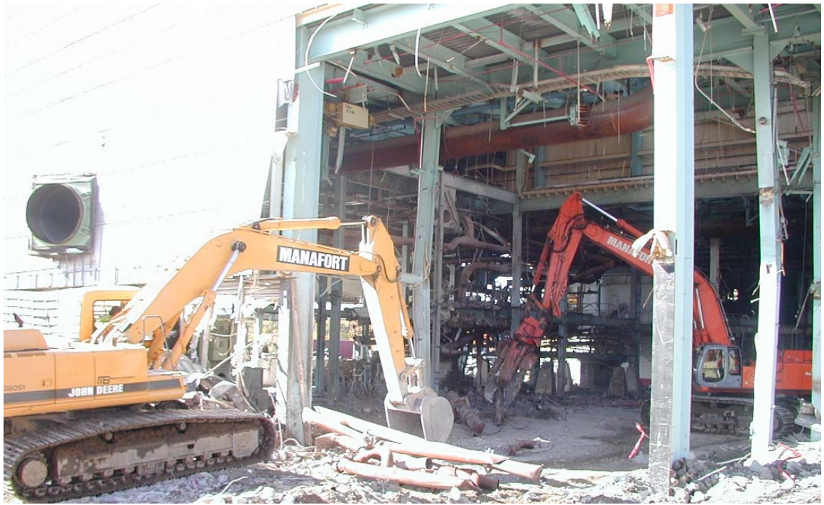
Figure A.4. Interior Building Mezzanine and Equipment Removal Prior to Demolishing the Structure
