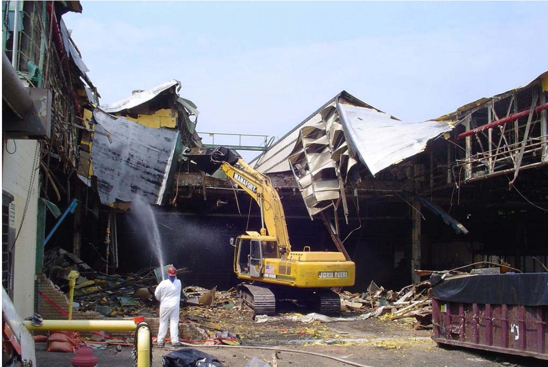
Figure A.3. Building Structure and Roof Demolition (Shear and Fugitive Dust Control)
